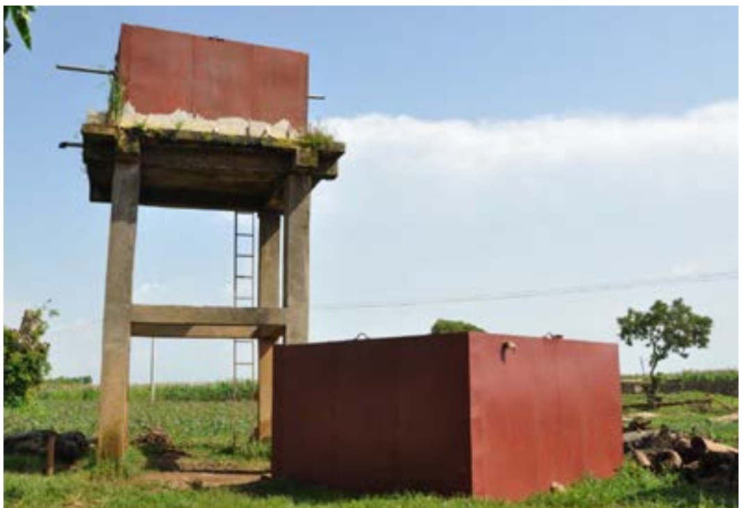
Figure A5.5. This water tanker was leaking and has been rusting for many years in Lalibela kebele, Amhara regional state. The one on the ground is a new tanker that will replace the old one
