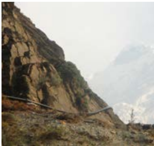
Pipe damage on steep slopes
