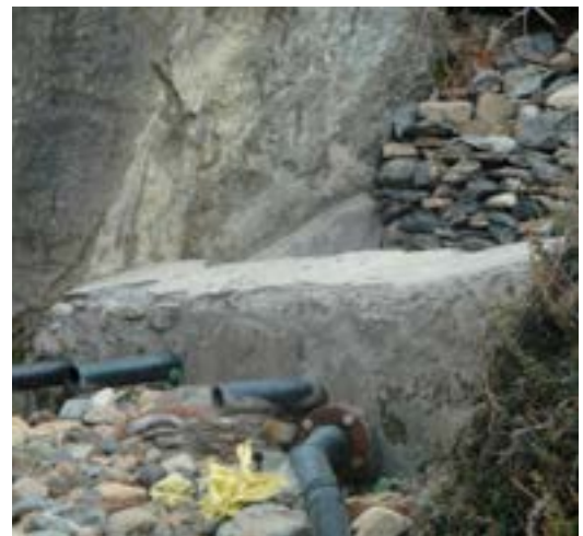
Due to groundwater depletion spring and associated intake structure is lower
