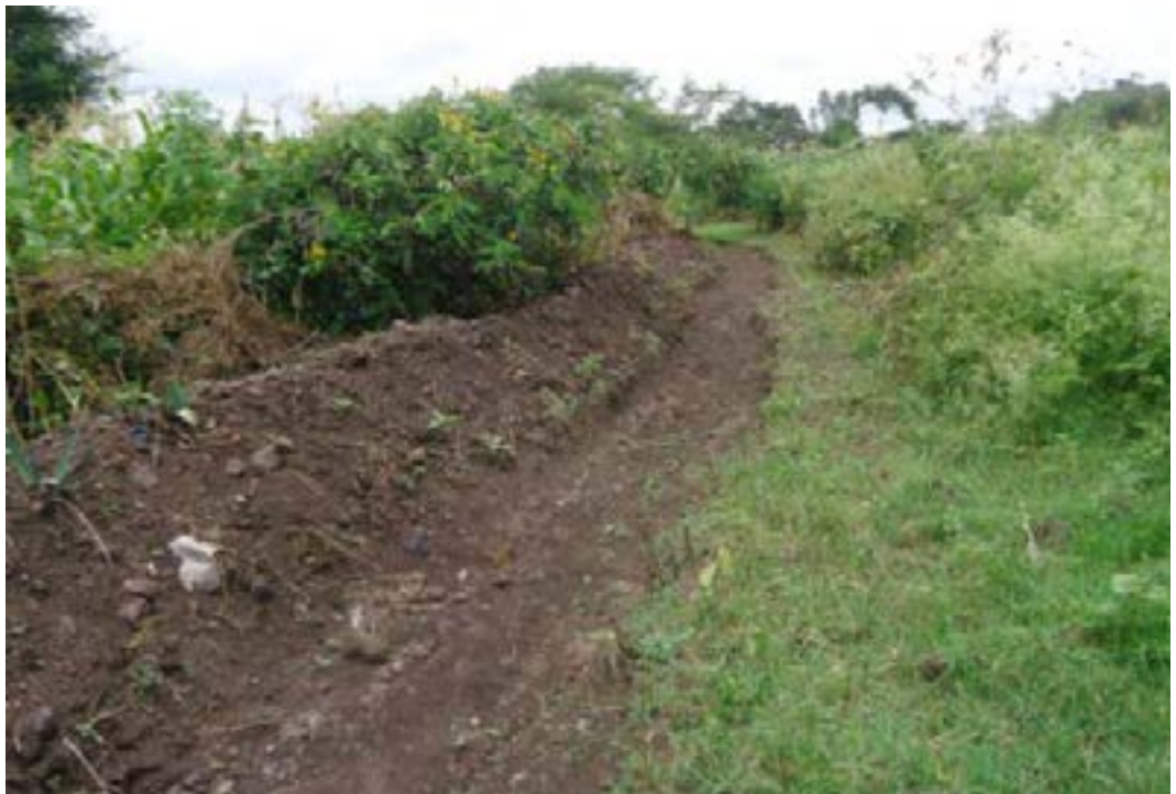
Figure A5.1. The community in Ellie kebele mobilized its own resources to dig a 250-metre diversion ditch to protect the only water source, which benefits more than 6000 people
