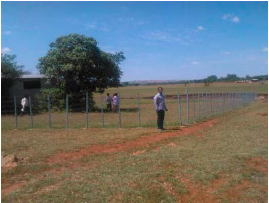
Figure A5.4. The community dug a diversion ditch and planted indigenous vegetation to protect the water scheme from potential flood damage and contamination. Proper fencing was also constructed
