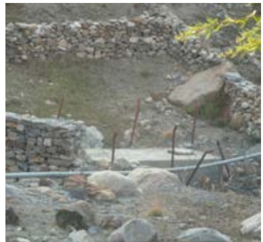
River intake prone to damage from landslide and flooding
