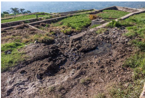
Damaged retaining walls and FS by-passing
