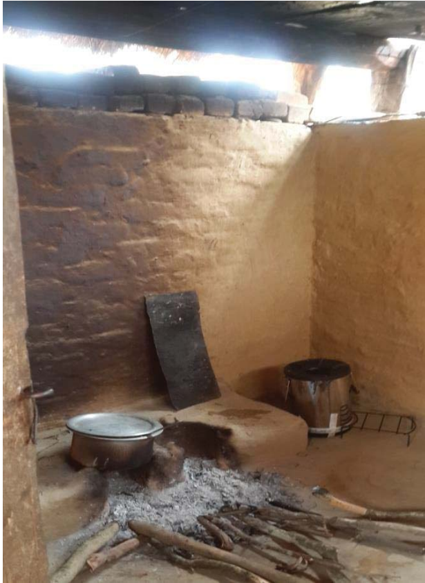
Figure 3. Kitchen with no window, some ventilation
