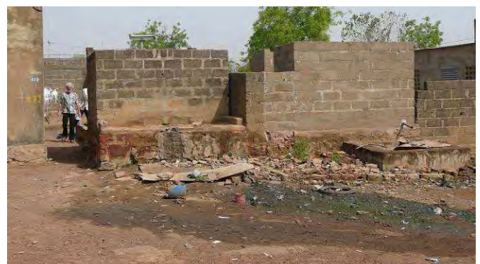
Fig. 8: Former desiccation (drying) chambers of UDDTs have been converted into pits to collect faeces and to be pumped empty when full (source: Stefan Hofstetter, March 2009).
