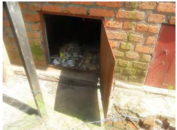
Fig. 10: Open vault of a UDDT in Kiziguro primary school. Paper is used as cleansing material.
