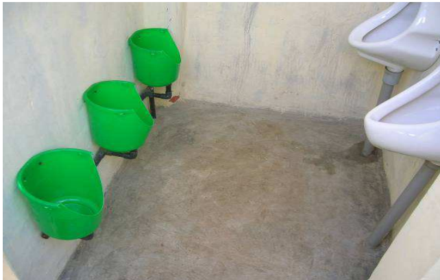
Figure 7 Inside the men's urinal showing the fabricated plastic containers urinal for the kids and standard ceramic urinals.
