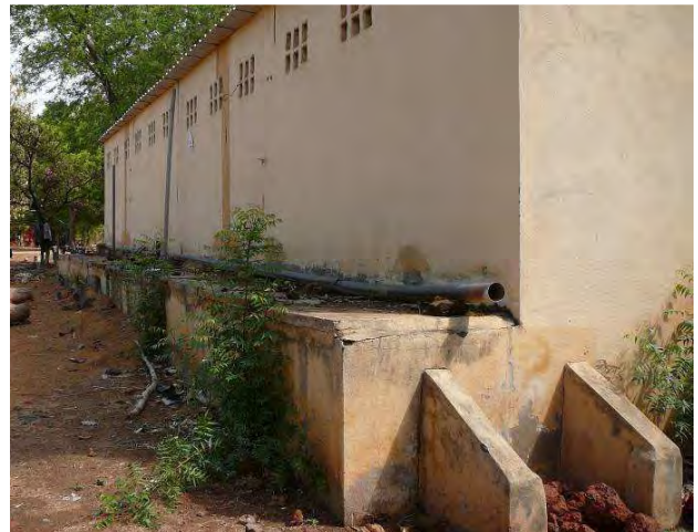
Fig. 10: Former urine collection of the toilet building at the school "Lycée du Séminaire Pie XII" (source: Stefan Hofstetter, March 2009).
