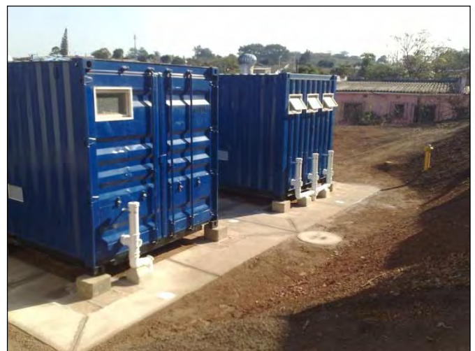
Fig. 3: Prefabricated container in Durban (source: eThekweni Water and Sanitation, 2010).
