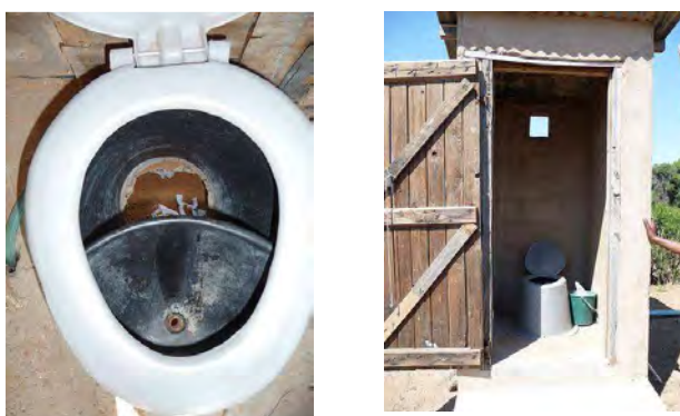
Fig. 7: Left: UDD toilet working properly in West Hanahai. Right: This UDDT was well maintained, ash standing next to the toilet and composting unit filled (in Paje).
