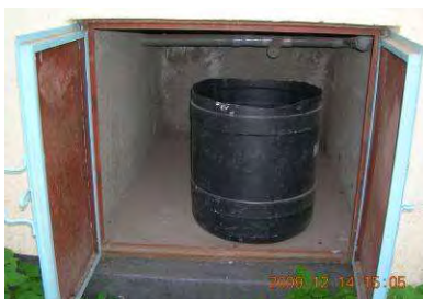
Figure 10 Interior of a faeces collection vault with a 50 litre container to collect the faeces (Source: Muchiri, 2009)
