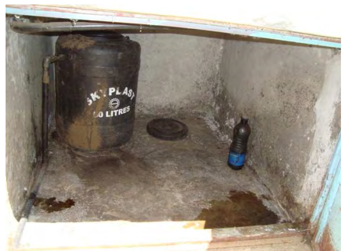
Figure 12 50 liter urine tank with small leakage in pipe (L.Kraft, May 2011)
