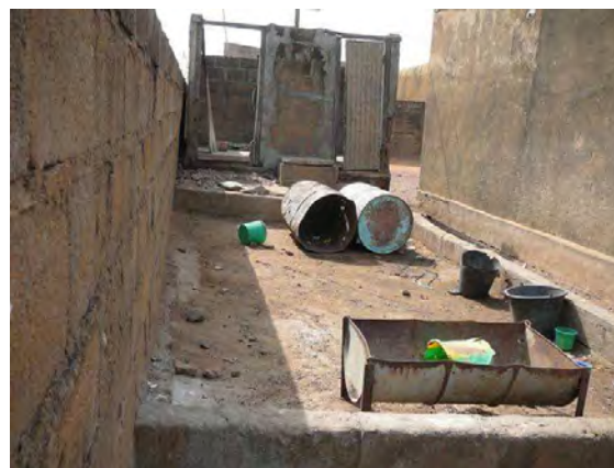
Fig. 7: A former greywater garden, which was once planted with lots of banana plants (source: Stefan Hofstetter, March 2009).
