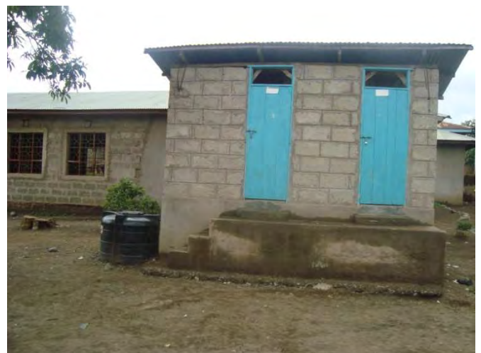
Fig. 3: UDDT toilet block (2 cubicles with 2 vaults each) made of concrete blocks in Daraja II primary school. The plastic tank for urine collection can be seen on the left side of the toilet. All pictures in this document are from the ROSA project in Arusha 2008-2010.
