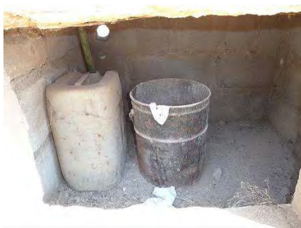
Fig. 6: Collection chamber under a properly working ecosan UDD toilet (left: urine container, right: faeces bucket) in Paje.
