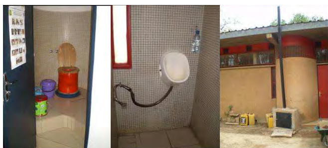
Fig. 6: UDDT inside a house (inside, backside view and waterless) (source: A. Fall, 2010).
