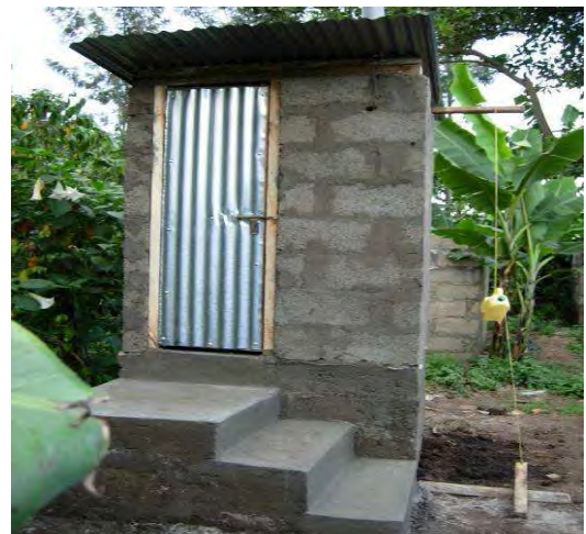
Fig. 5 Single vault UDDTs in Daraja II built with concrete blocks (source: ROSA, 2008).
