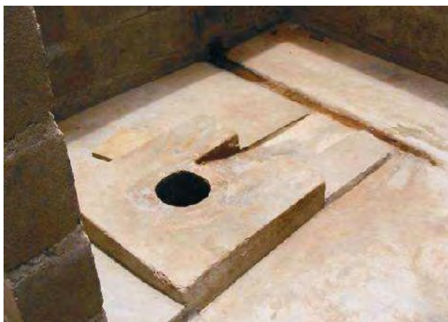
Fig. 6: Latrine urine-diversion squatting pan, where urine drains away to the drainage at the right (source: GIZ, 2002).
