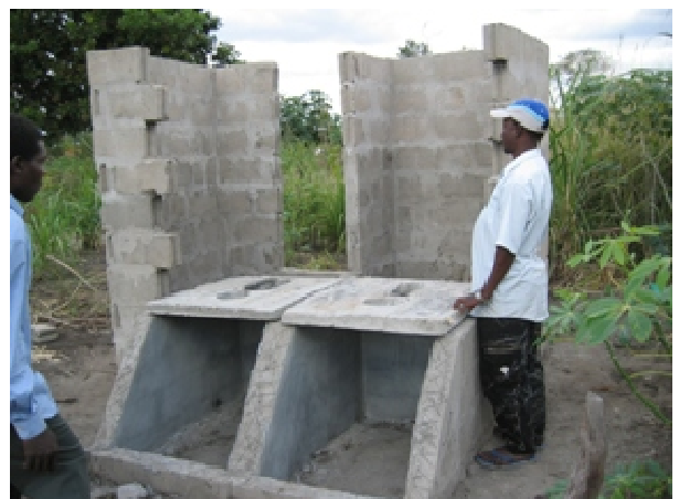
Fig. 4: Construction of a double vault UDDT in 2003; the two faeces vaults are visible at the front (source: M. Fogde, 2003).
