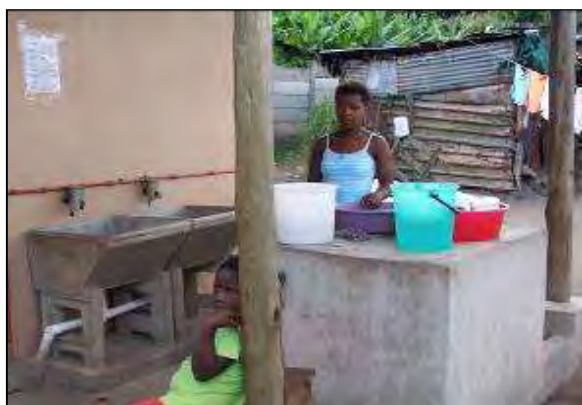
Fig. 7: Examples of washbasins and laundry facilities at CABs (source: EWS, 2008).
