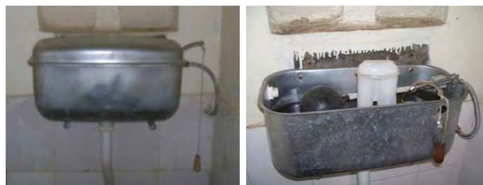
Fig. 13: Cistern after installation (left) and after vandalism/misuse and theft (right) a few weeks later. Repairs were undertaken by WSP, but the toilet operator now shifted to a pour flush system.
