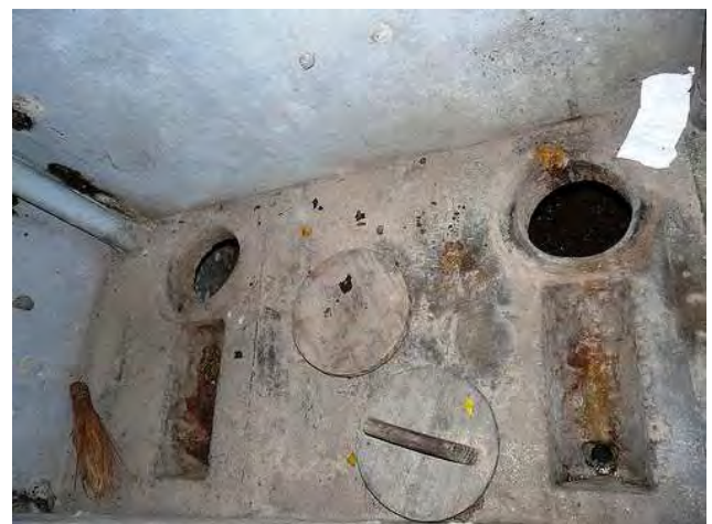
Fig. 6: Very dirty and not well maintained UDDT (inside), 8 years after construction. It seems that both faeces vaults are used at the same time. Note the two round wooden lids to cover the faeces holes (source: A. Leitner, 2011).
