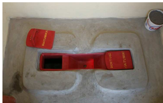
Fig. 8: Inside view of a UDDT with ash container on the right. The squatting pan has two faeces outlets: only the one on the left is currently in use. In the left corner is the ventilation pipe (not visible) (source: Moses Wakala, GIZ-Kenya, June 2008).
