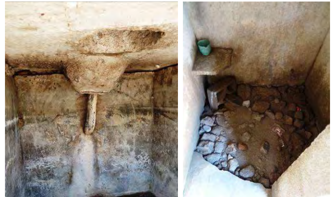
Fig. 9: Situation 8 years after construction: Left: walls of faeces vault with deep cracks. Right: bathing cubicle's concrete floor is broken (source: A. Leitner, 2011).
