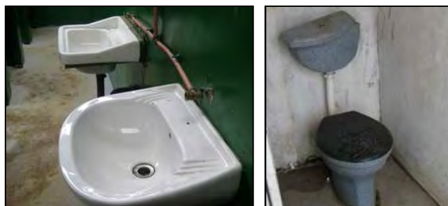
Fig. 8: Interior of CAB (Left) and flush toilet in CAB (Right) (source: Roma, 2010).
