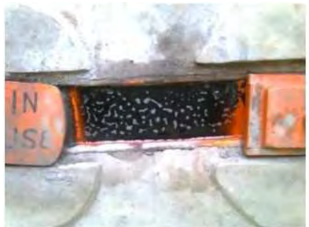
Fig. 11 A urine pipe got blocked with ash at Muslim Primary School, Mumias (Source: Laura Kraft, GTZ, June 2010)
