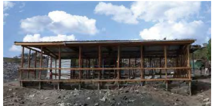
Fig. 11 Drying shed at the dump site for centralized composting (source: Sustainable sanitation Practice, Issue2. 01/2010, EcoSan Club)
