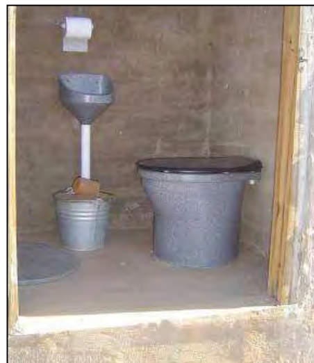
Fig. 9: Inside view of UDDT: urinal for men (left), bucket containing sand or ash and cover over second vault on the left side, as well as urine diversion pedestal to the right (source: EWS).
