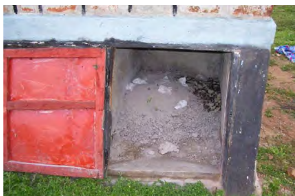
Fig. 7: Faeces collection vault which is half full (source: David Watako, GIZ-Kenya, July 2009). Note: Sufficient use of ash
