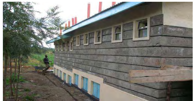
Figure 11 Ventilation pipes and windows for each UDDT collection vault and cubicle respectively (Source: Muchiri, 2009)
