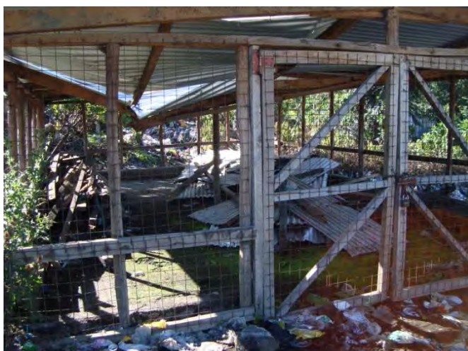
Fig. 13 Drying shed was destroyed during a storm (Source: L. Kraft, May 2011)
