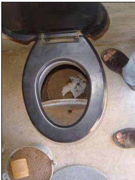
Fig. 10: Interior of a UDDT with sand container on the bottom left and plastic urine diversion pedestal at the top from Atlas (source: EWS)
