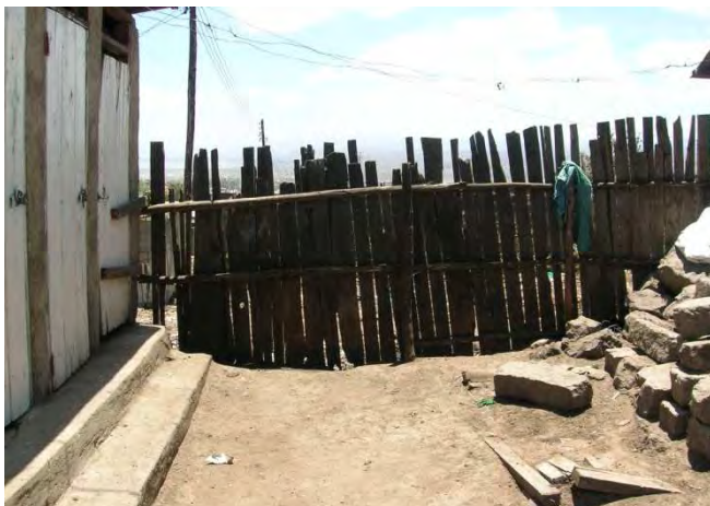
Fig. 5 Existing pit latrines (left) and a buried filled up pit latrine in the front on which the new UDDT was constructed
