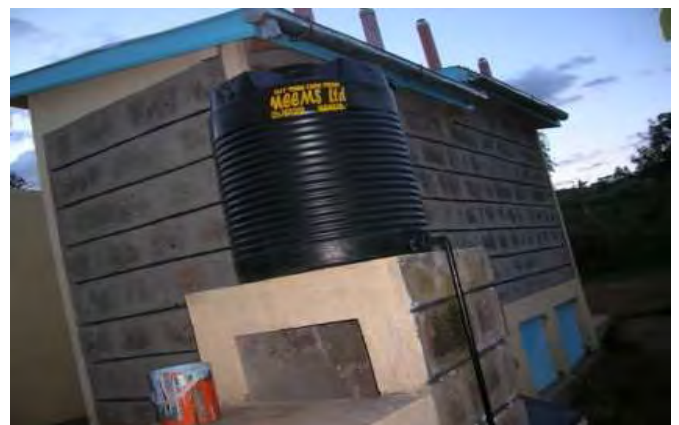
Figure 8 Roof water harvesting system for hand washing at the new UDDT.
