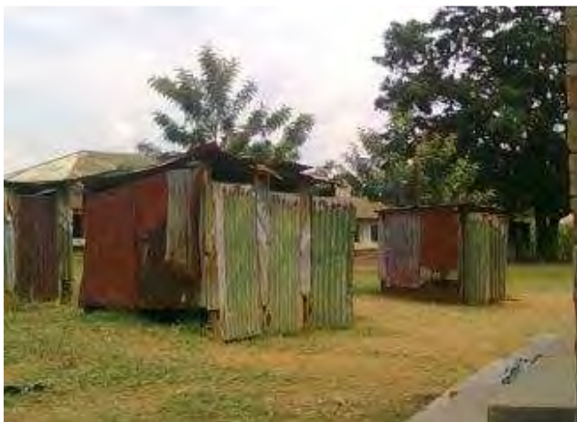
Fig. 4 Old pit latrines at Muslim Primary School, Mumias (Source: Laura Kraft, GTZ, June 2010)
