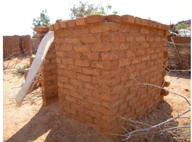
Fig. 4: Superstructure of a double pit latrine. Is this the material usually used for the superstructure? Fig. 7 indicates a much simpler version. Do the pit latrines not have a roof? Why? What about privacy or similar issues? (Source: J. Patinet (2009) Groupe URD).
