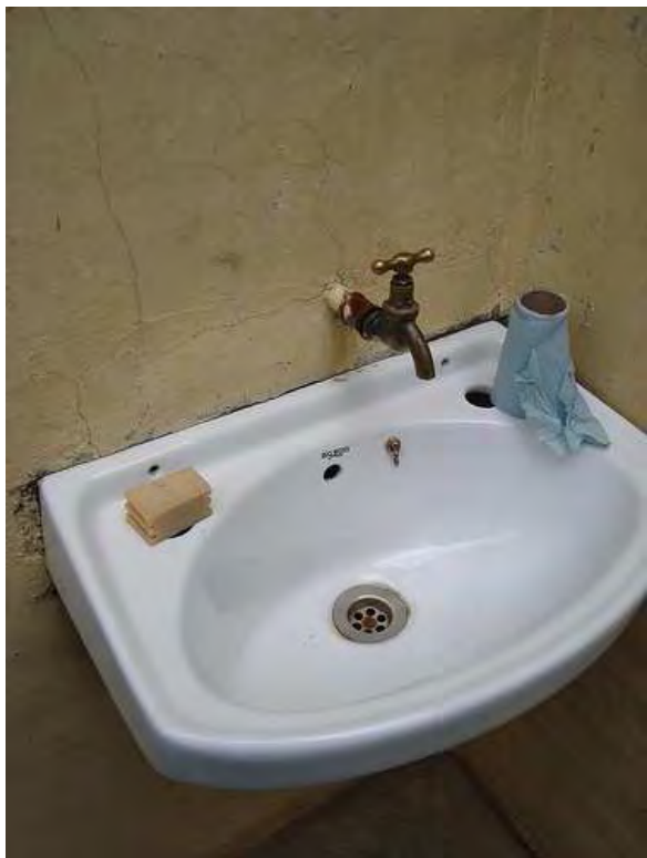
Figure 16 Handwash facility was in good conditions. Toilet paper and soap is provided by the school Source: L. Kraft, May 2011)
