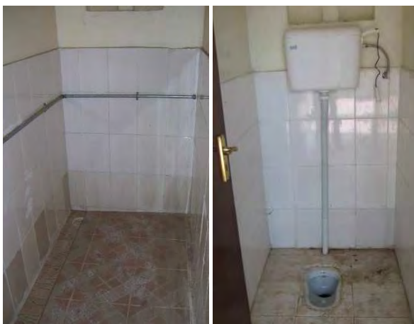
Fig. 6: Left: Urinal using a tiled wall (no door) with optional water flush. Right: Squatting pan with 10 L cistern (flush toilet); but these days a manual pour flush system is used for toilet flushing (see Fig.7).
