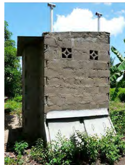
Fig. 12: Household UDDT in good condition, 8 years after construction; note metal faeces vault covers are still in place (source: A. Leitner, 2011).
