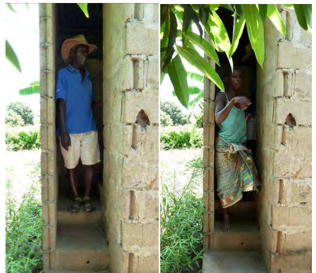
Fig. 10: The entrance to the UDDTs is very narrow (source A. Leitner, 2011).
