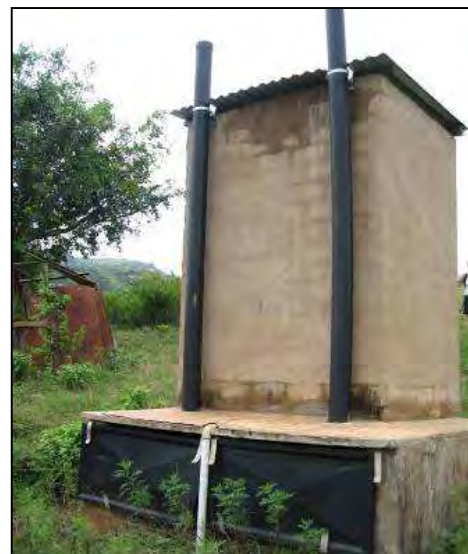
Fig. 6: UDDT back view showing access doors to two vaults and ventilation pipes (source: EWS).
