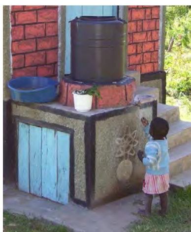
Fig. 12: Hand wash facility with 100 litre tank and tap secured in concrete located on top of urine tank storage vault (Source: Moses Wakala, GIZ-Kenya, Jan. 2010).
