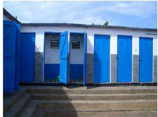
Fig. 4: New students' toilets (45 UDDTs) - these are now five years old and still in perfect condition (source: EcoSan Club, 2009).
