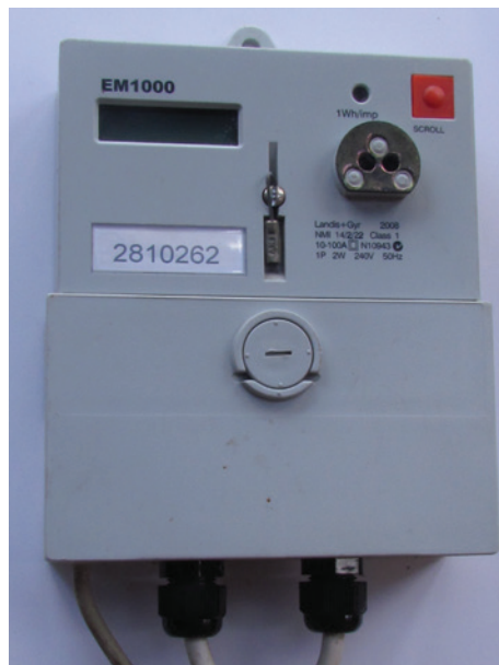
Figure 4.5 Electricity meter attached to data logger setup (for demonstration purposes only).
