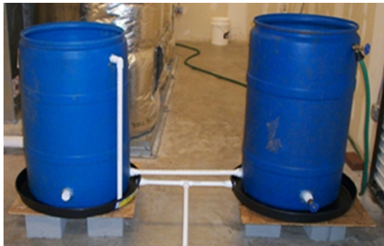
Figure 9.8 Condensate holding tanks and irrigation pump.
