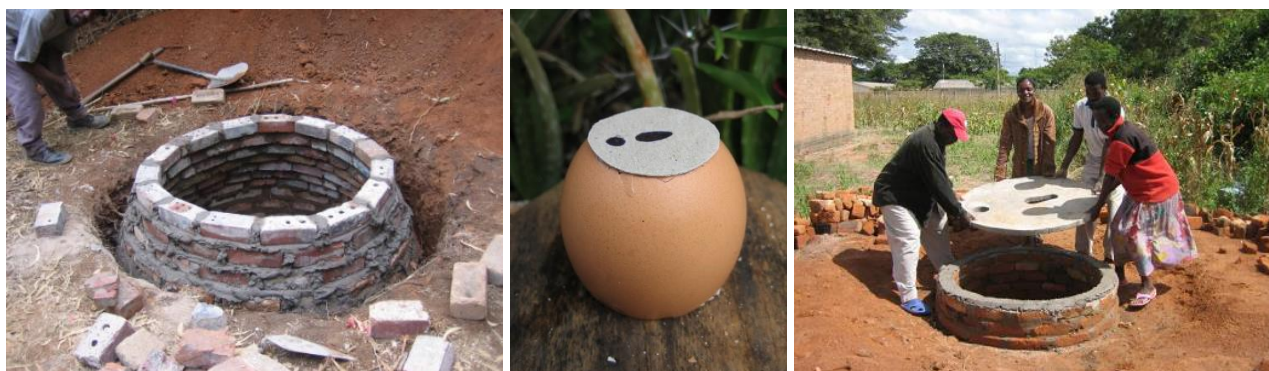
Modern Blair VIPs are built with a conical (corbelled) brick pit lining which gives the pit lining great strength.
