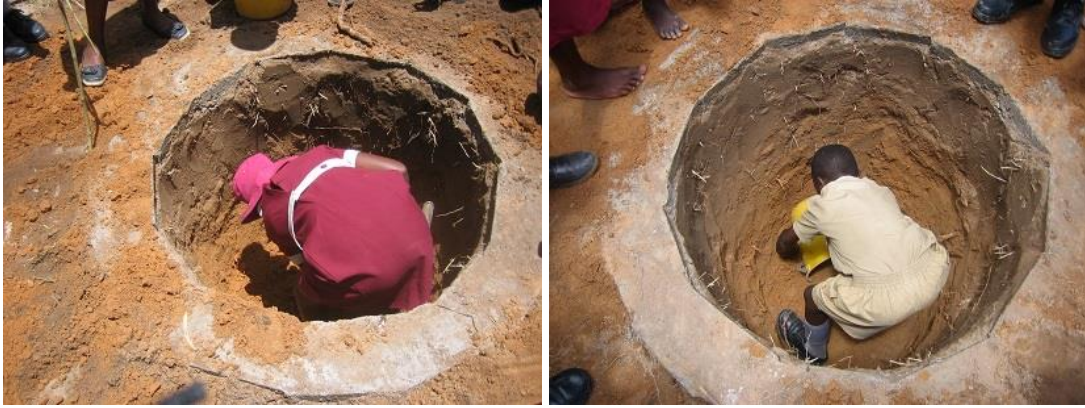
School children digging the pit of an Arborloo at Chisungu Primary School, near Harare.
