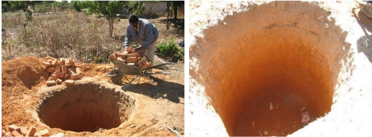
The pit is dug 1.7m wide and 2m deep. Walls are straight and bottom flat
