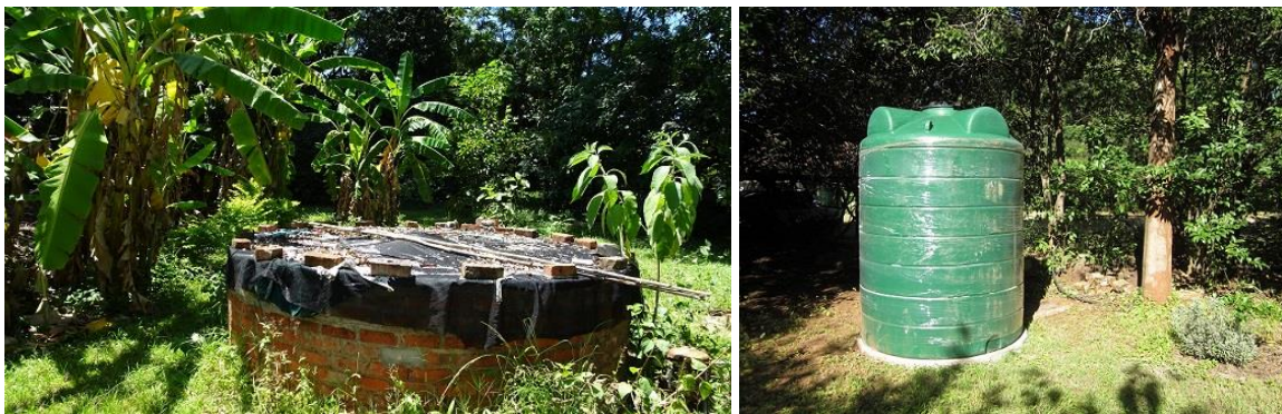
A brick built storage tank with heavy duty plastic and shade cloth cover. A 5000li plastic tank
