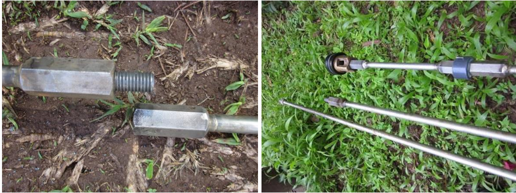
12mm stainless steel rod connector and the rods prepared for lowering down the rising main.
