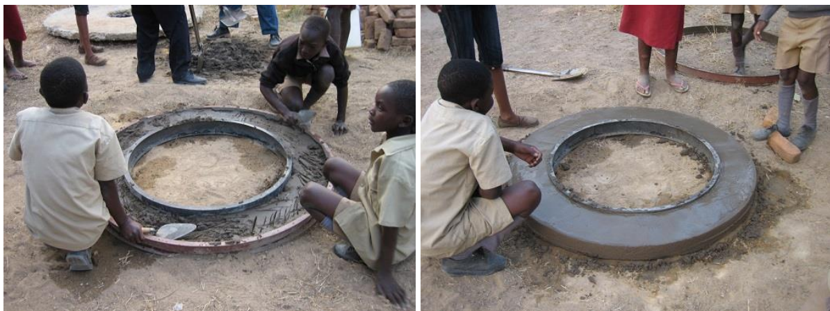
A steel ring beam mould is being used to make the ring beam
