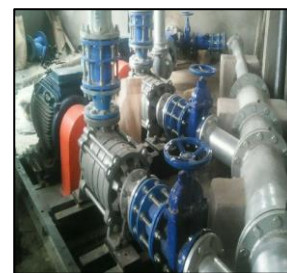
Picture 2: Production borehole pumping station, Wukro
