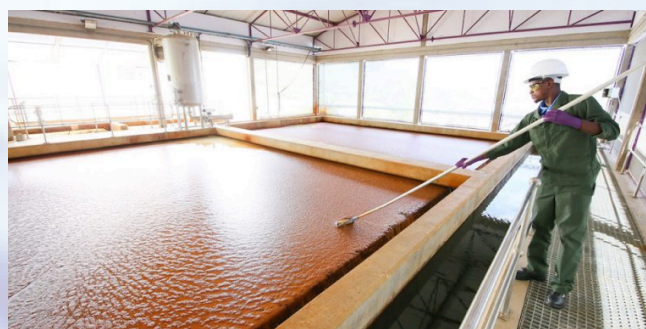
Photo: Windhoek Wastewater Treatment Plant, Credit Photo : Afrik 21
