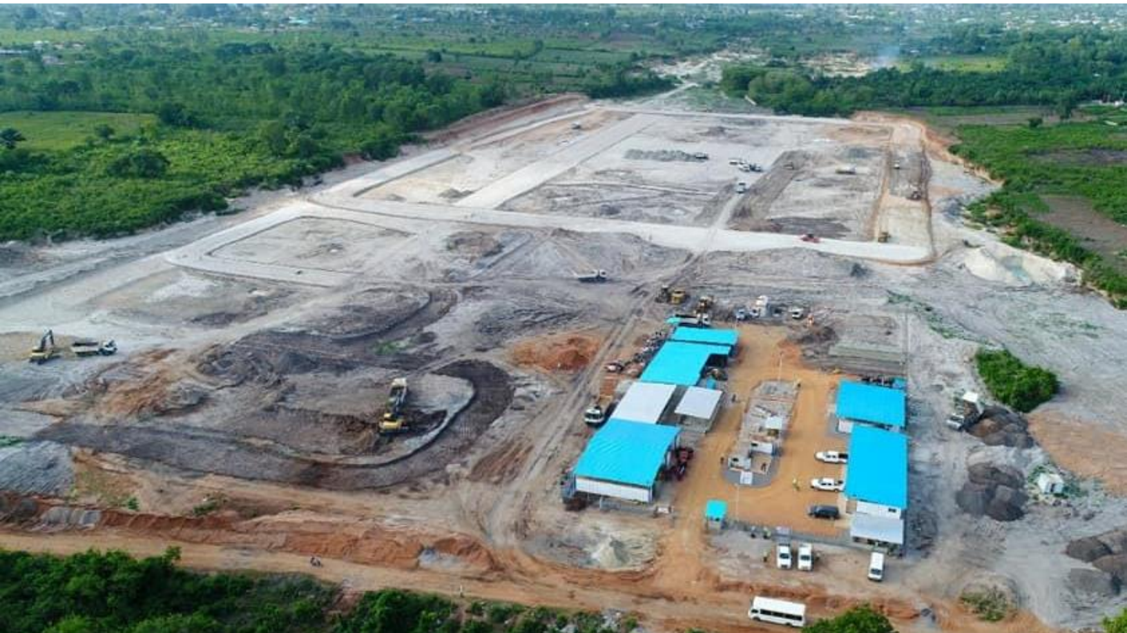
CALAVI- BENIN SLUDGE TREATMENT PLANT (STBV) © SONEB 2018
