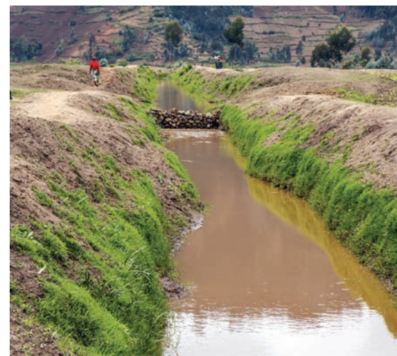
Storm water drainage is a key part of wastewater management
