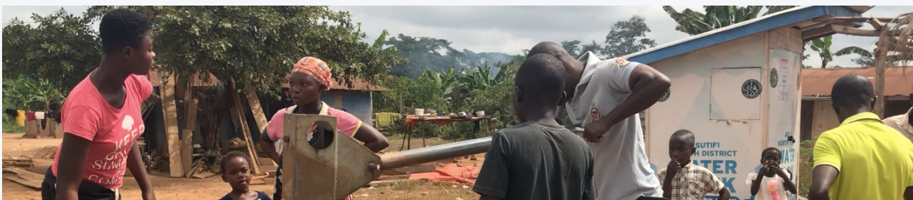
Image 1. A technician works to repair a handpump next to a kiosk in a rural community in Asutifi North.
