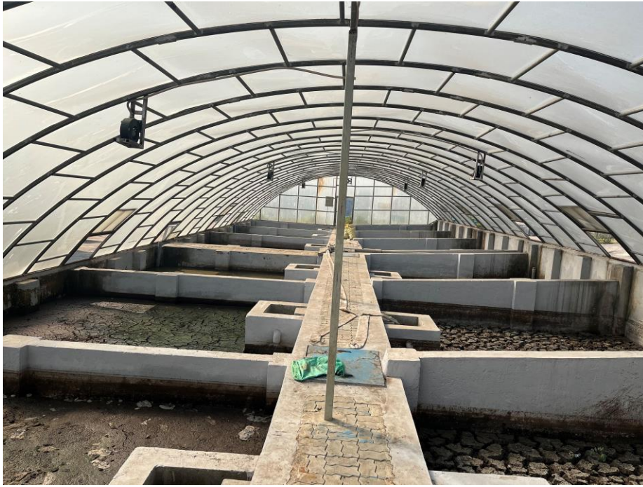
Figure 2: Sludge drying beds with Greenhouse Solar Dryers (GHSD), Angul FSTP
