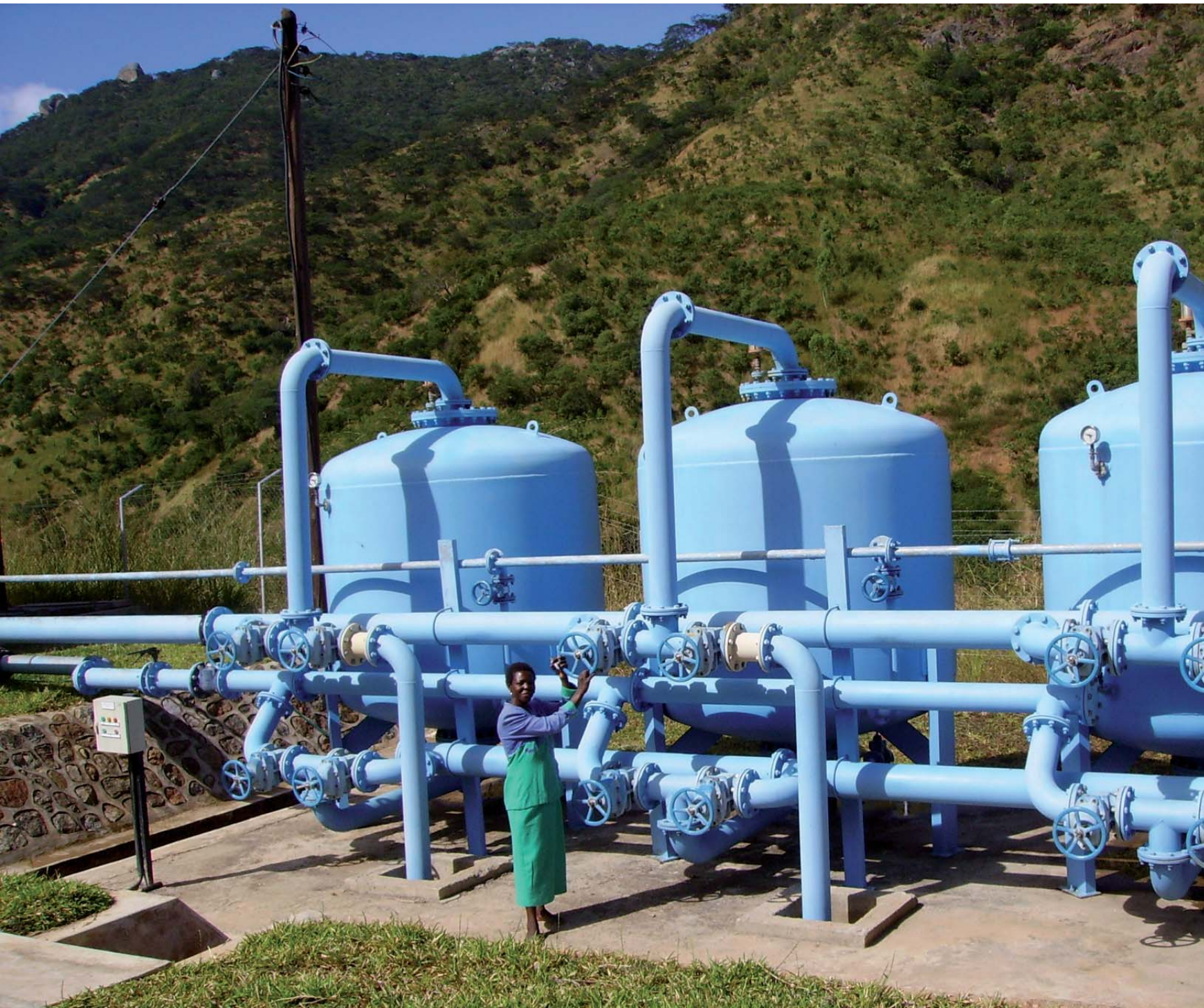
Operator at a water treatment plant in Rumphi, Malawi
