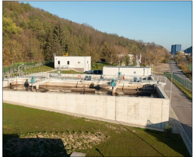
Figure 13: Optimized engineering in sewage plants – Biogest International GmbH equips a sewage treatment plant in Provadia, Bulgaria
