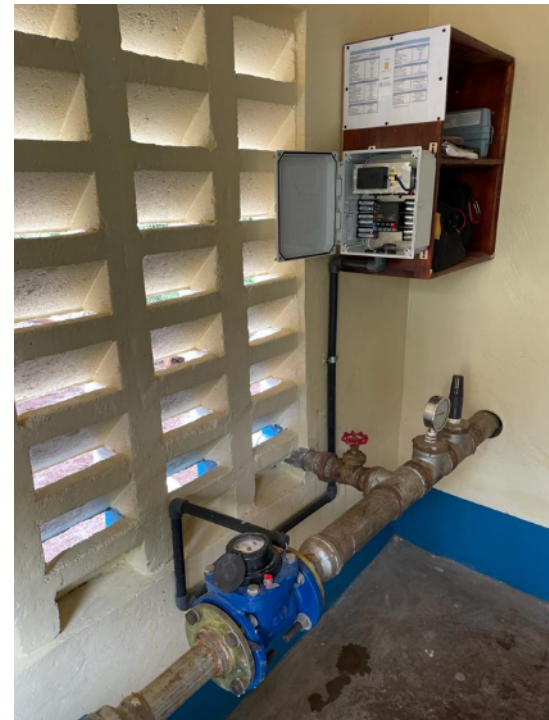
Figure 19. Water Mission SatWater Communicator connected to a pulse water meter in a pumphouse (Source: Water Mission)
